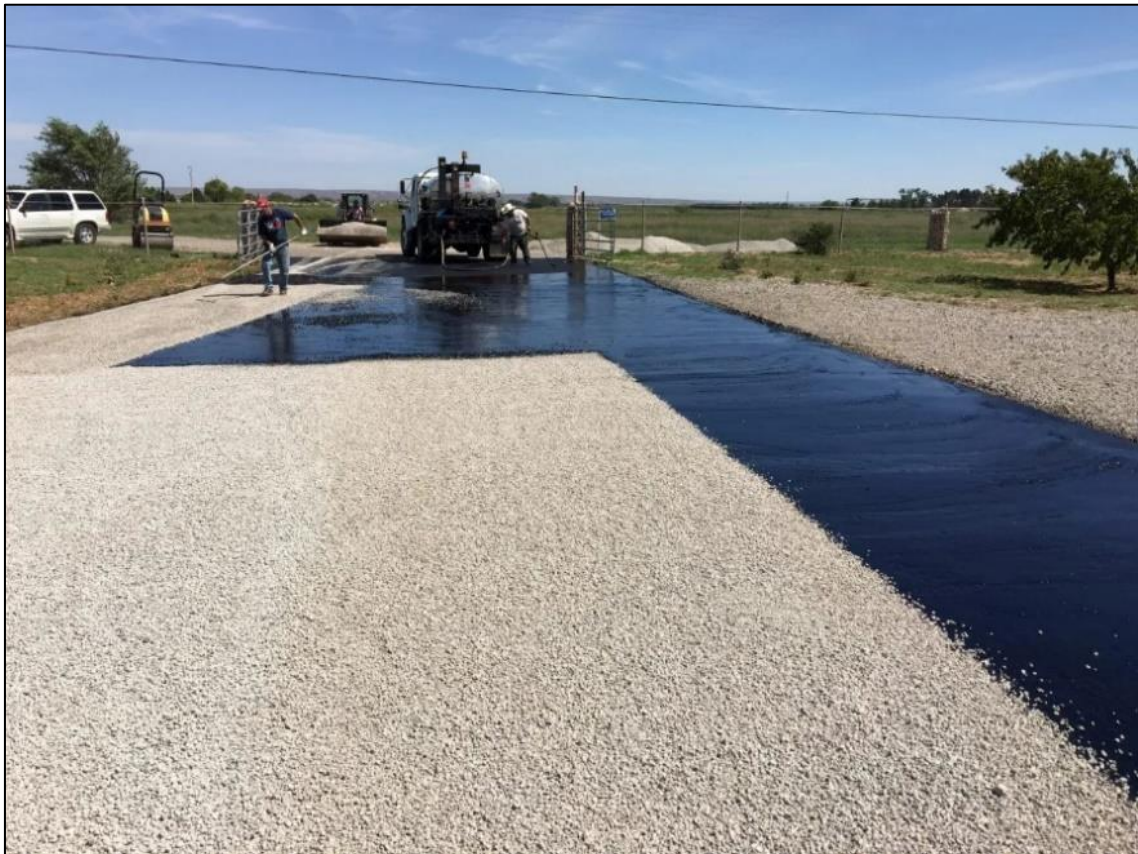
Figure 4. 7: Application of Chip Seal on a low-volume rural road (Reference: Driveway Experts )
