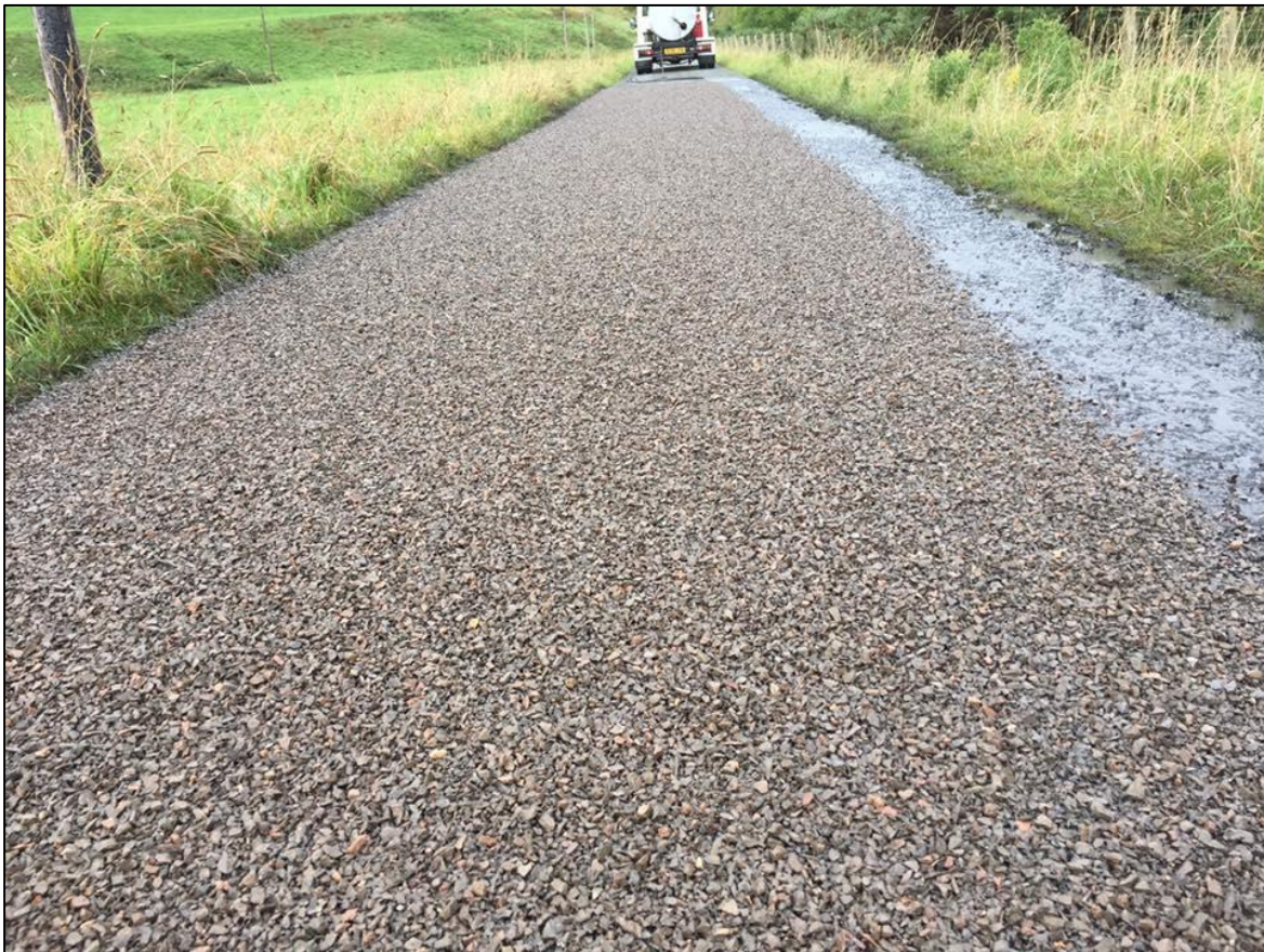
Figure 4. 11: Application of a Surface dressing low-volume rural road (Reference : Colas (top) and Northumberland Surfacing (bottom))
